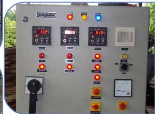
Control Panel For Automatic Operation
