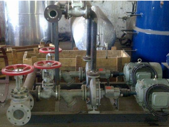
2 Nos. Circulating Pump Assy.
